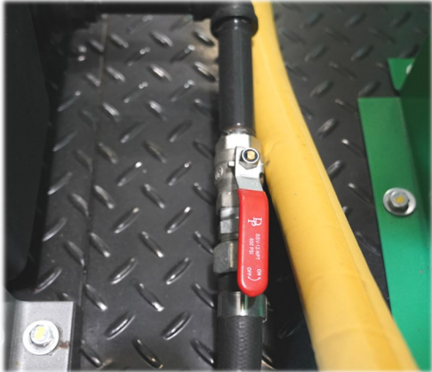
Figure 6. Valve is pictured in the open position
