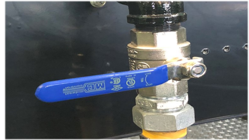
Figure 7. Valve is pictured in the closed position
